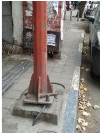
Photo 16 Electric Pole on Footpath at Bajirao Road
