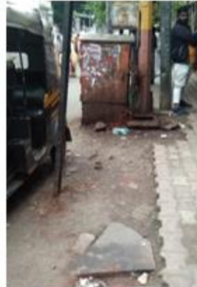
Photo 13 Broken Footpath on Shivaji Road
